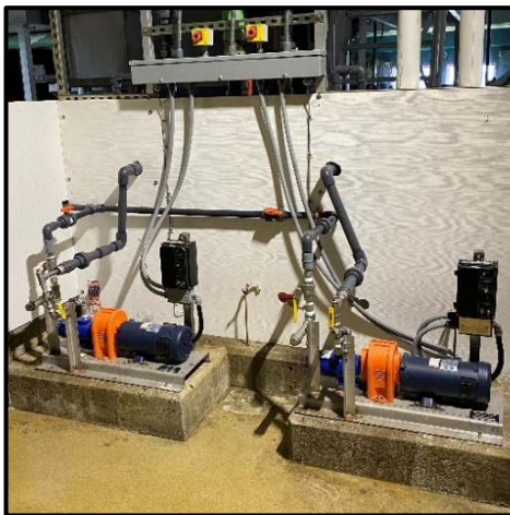
PBU 1 & 2 Installed and in service.
